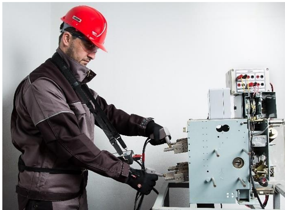
Figure 3-3: Connecting RMO-H to circuit breaker using cables with Kelvin probes
