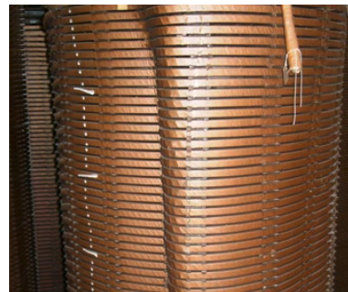
Buckling of winding
