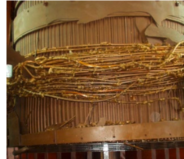
Collapsed tap winding
