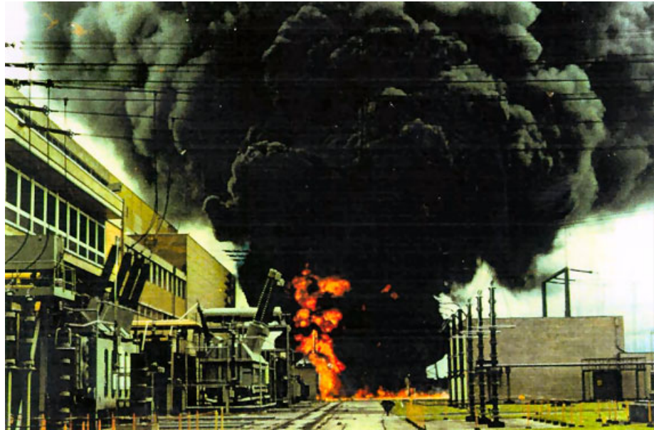
Figure 12-6 Transformer fault due to a defective bushing
