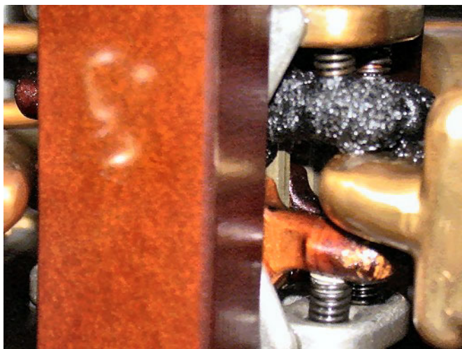
Figure 12-17 Bad tap selector
